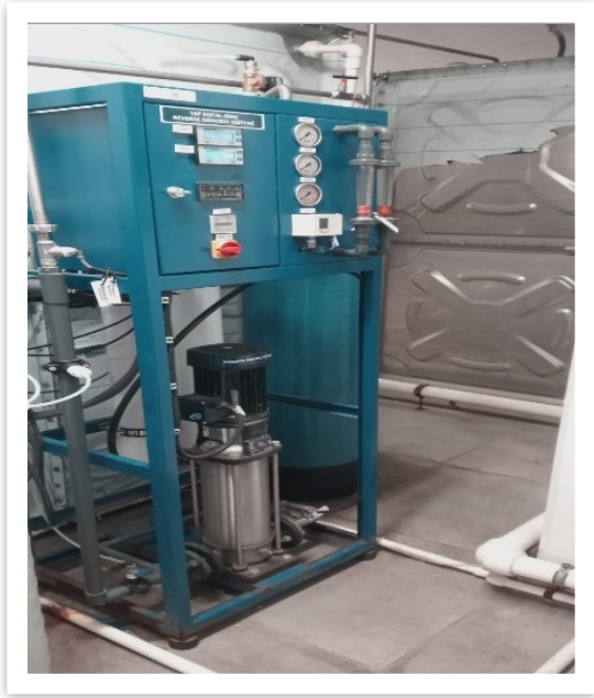
Reverse osmosis system
