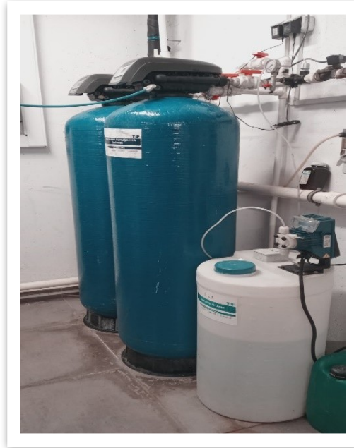
Water softening system
